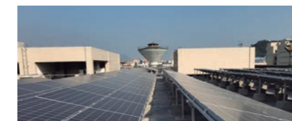
Solar power generation facilities are in operation at manufacturing bases in Japan, China and Thailand
